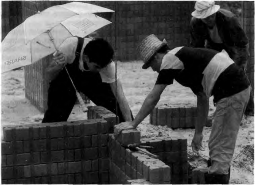
Self help in construction: The project of Ubon Ratchathani, Thailand A new laminated brick is being used
