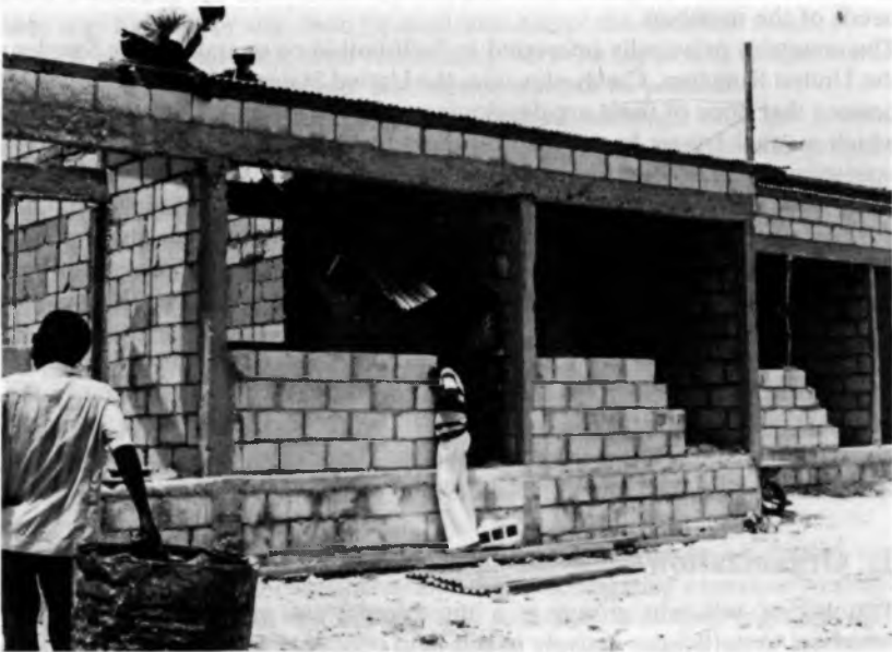
Project in Port-au-Prince, Haiti of the San Martin Housing Cooperative Foto: CHF
