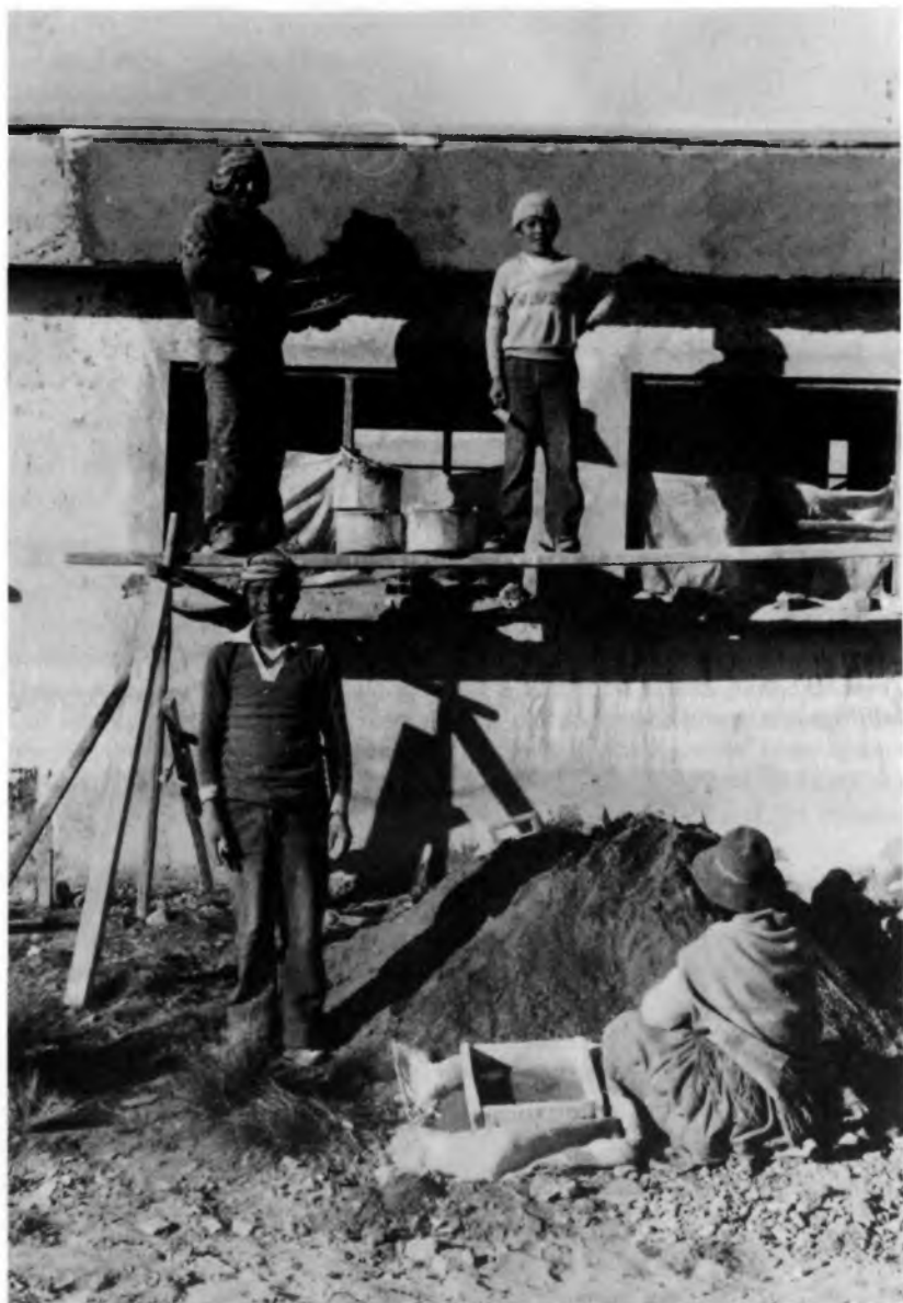
Members carry out the final work of the project "El Alto" in Bolivia Their families will have a better home . . .
