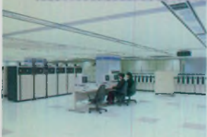
Ishioka Center Computer room
