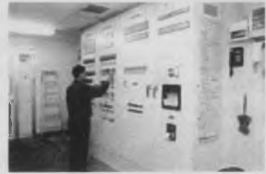
Machine room to control operation
