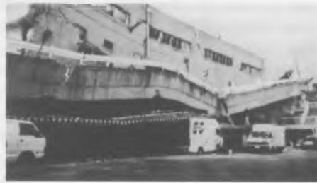
Collapsed Co-op Living Centre
