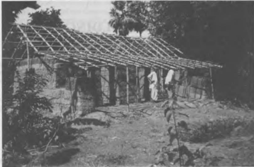
Mud houses in West Bengal, India Monetary input per house: 250, – US-Dollar (tiles, doors, windows) Carcass of mud houses
