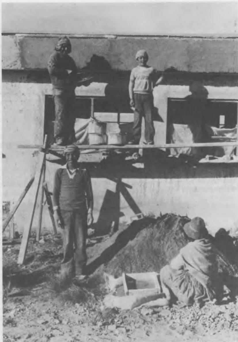
Members carry out the final work of the project "El Alto" in Bolivia Foto: DESWOS Their families will have a better home . . .
