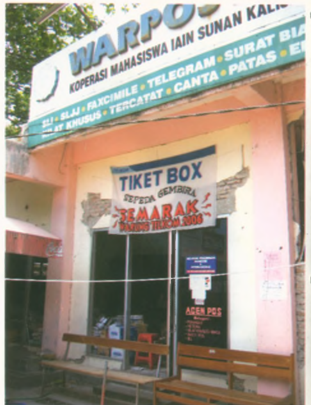
A view of the damaged store
