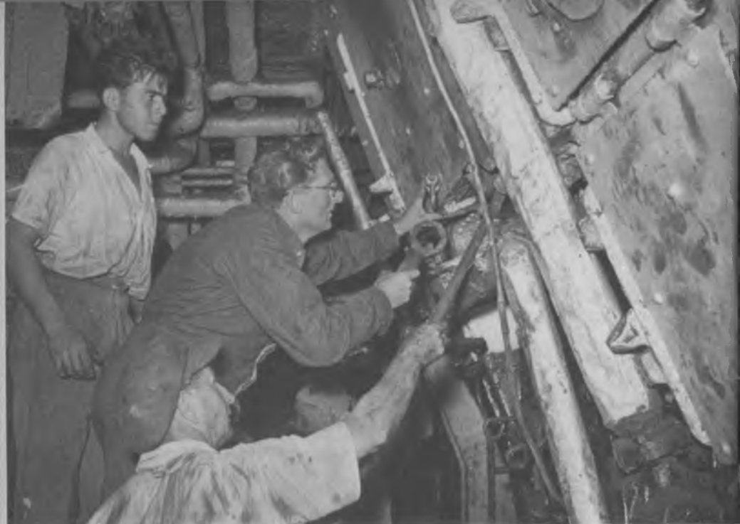
The repair and restoration of the co-operative ship Agur in the Port of Haifa.
